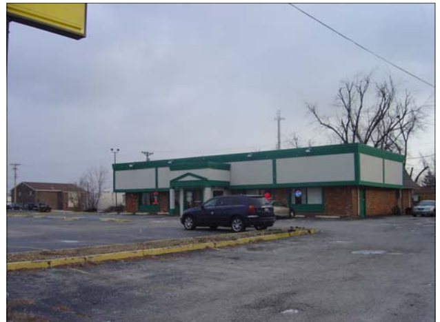
This parking lot for Fortel's Pizza Den is severely deteriorated.
