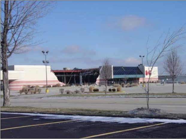
The vacant K&G store has severe storm damage.
