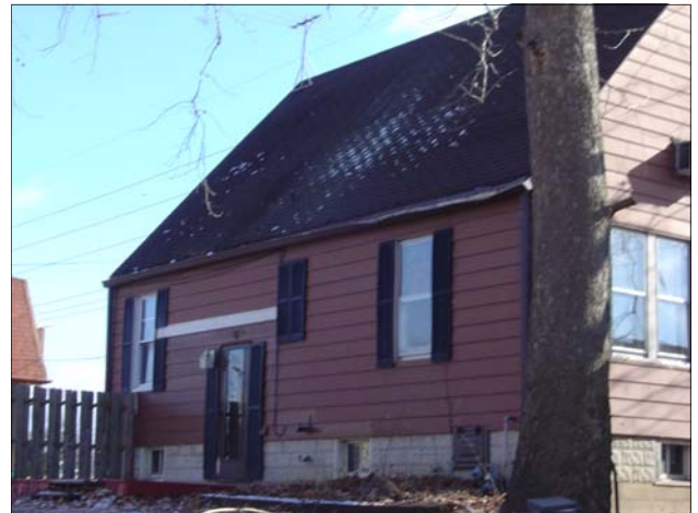
This gutter on this single-family is sagging badly and there is a missing section of shutter where the siding was replaced.
