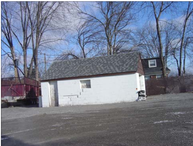
This accessory structure for the Fix-O-Flat has severe step cracking and the wall is falling inward.
