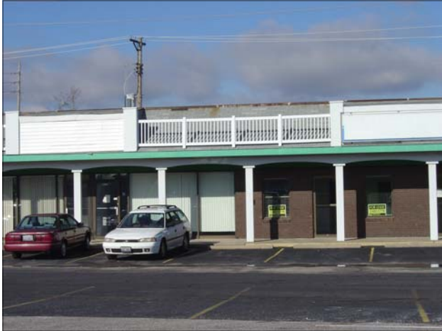
This strip mall along Lincoln Trail contains several vacancies. Note roof cap is rusting.
