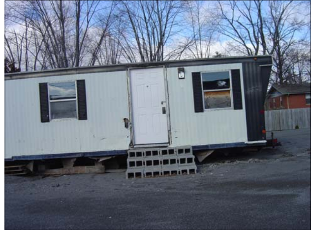
This mobile home behind the Fix-O-Flat is severely deteriorated and has tires stored in and around it.
