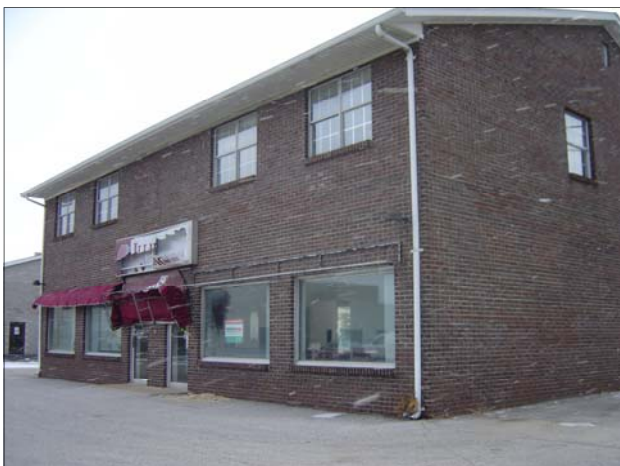
The signage and awning on the front of this vacant commercial building fronting Canty are broken and missing sections.
