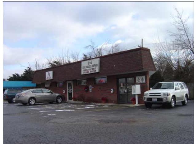
The parking lot for this multi-tenant commercial building is cracked and crumbling.
