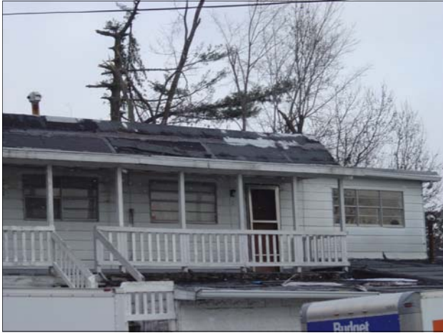
The roof on Fairview Sports & Hardware is sagging and has no shingles.
