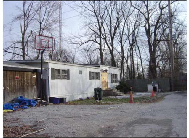
This mobile home fronting Voss is dilapidated and has been declared unsafe for human occupancy by the City.
