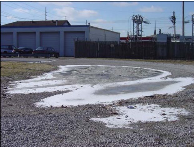
The parking lot in the rear of Screamin' Demon Tattoo is severely deteriorated and contains large puddles of water.
