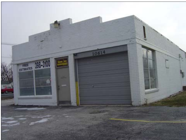
This former body shop is now vacant. Note step cracking on the front and sides of the building.
