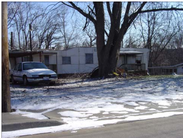
This mobile home fronting Ruby is deteriorated. Note large branches on carport roof.
